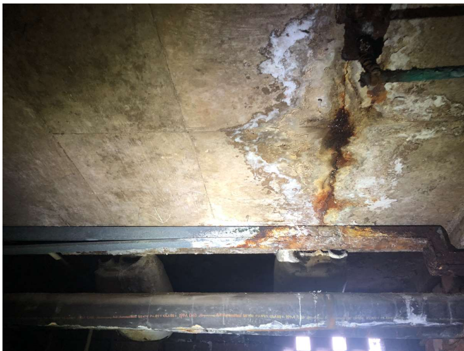
Photo 26: Underside of floor shown in photo 13. Pool water is penetrating the concrete floor causing corrosion of the reinforcement and staining of the soffit.
