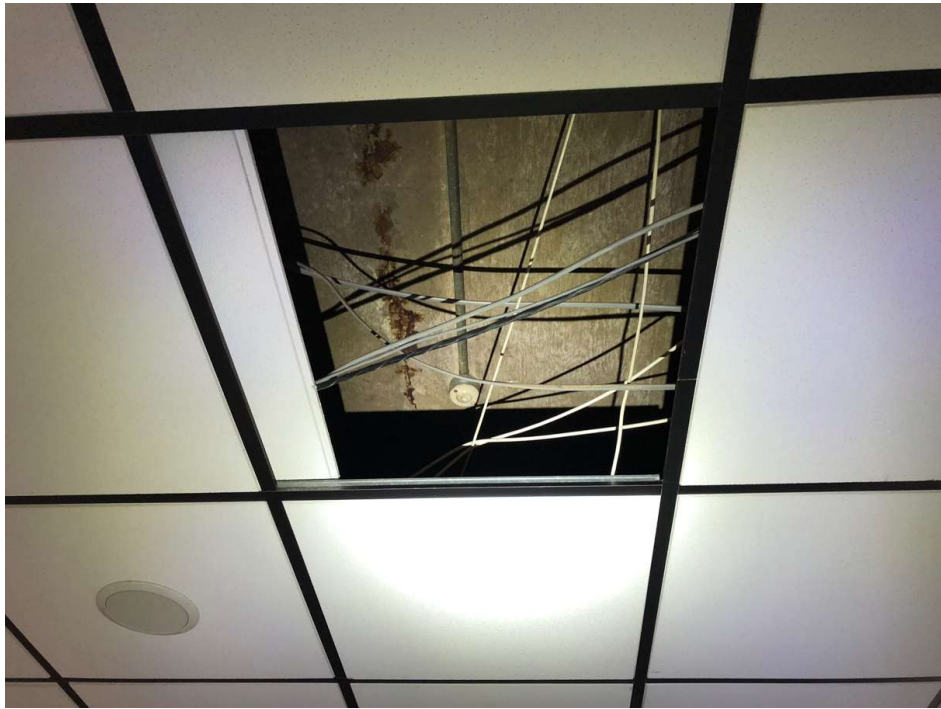
Photo 35: Underside of concrete roof slab, first floor corridor outside the changing rooms. Staining indicates corroding reinforcement due to leaking flat roof finishes above.
