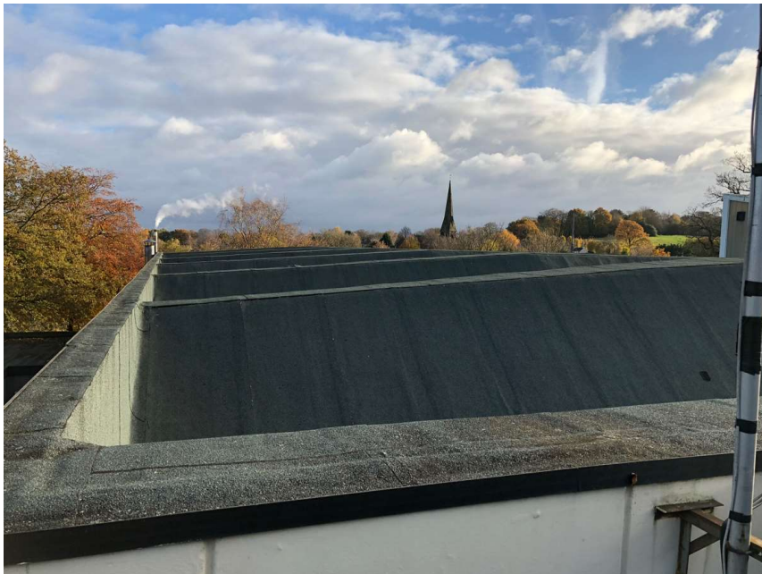
Photo 42: Roof over Main Pool. Structure projecting above. Felt looks in reasonable condition to this part of the building.
