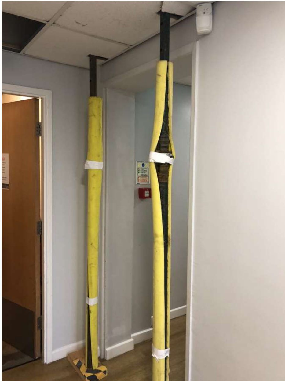
Photo 55: Since our original survey the RAAC panel has been temporarily propped as a short term 'make safe' precaution.
