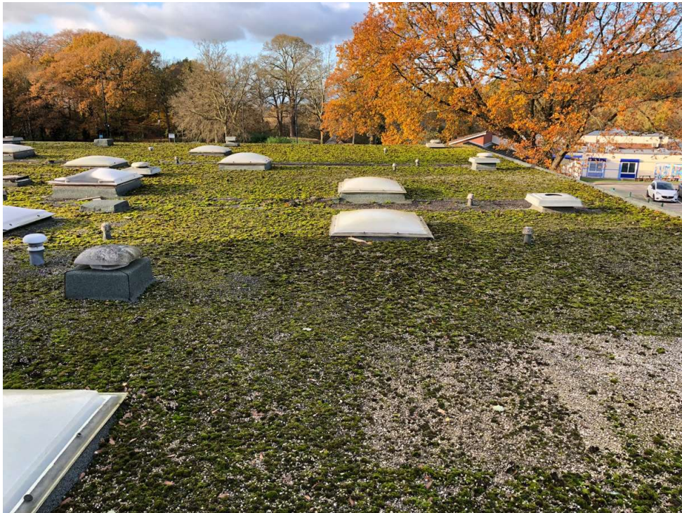
Photo 39: Flat roof over main entrance and Spa area. Heavily vegetated. The felt is in poor condition.
