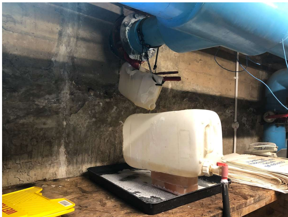
Photo 30: An interesting way of catching the leaks.
