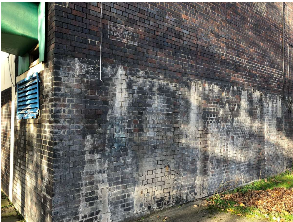
Photo 8: South corner. Stained brickwork, but the cause could not be determined. The swimming pool tank basement area is behind this wall.
