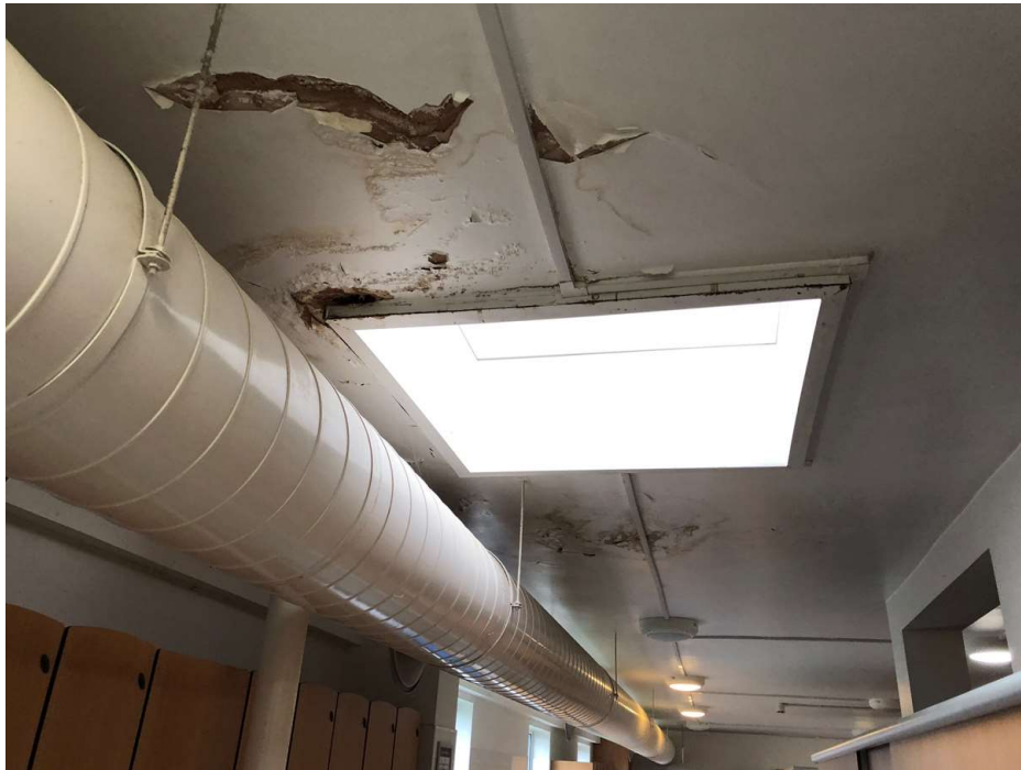
Photo 21: Extensive water damage due to the leaking flat roof over the changing rooms.
