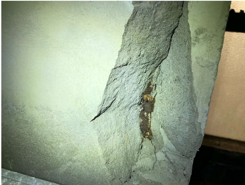
Photo 25: Corroding, expanding, steel reinforcement within the column causing the repair to fail.
