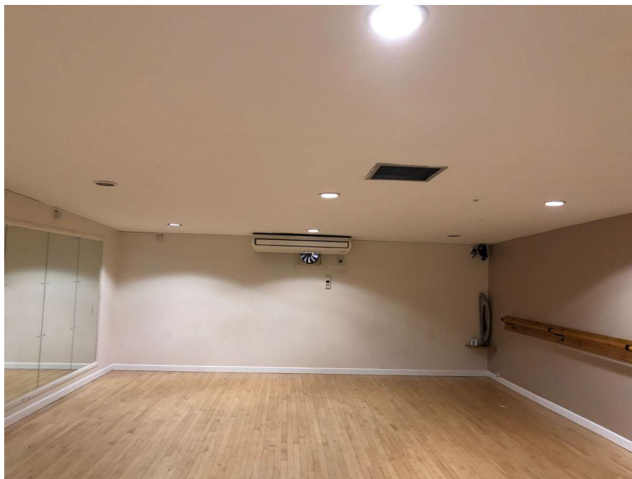
Photo 55: Internal view of dance studio at first floor. There are RAAC panels above the solid plastered ceiling. Condition of RAAC unknown.
