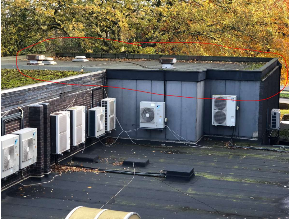
Photo 50: Roof of RAAC building. Laid to a fall towards the far end. The felt appears to be in reasonable condition. The grey vertical wall panels are RAAC.
