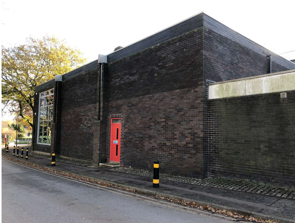
Photo 41: Northeast elevation of fitness suite. Brickwork cavity wall is in reasonable condition.
