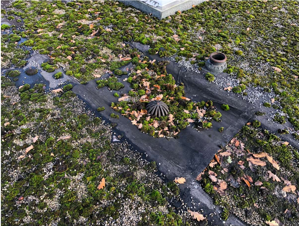
Photo 41: Failing roof felt and drainage.
