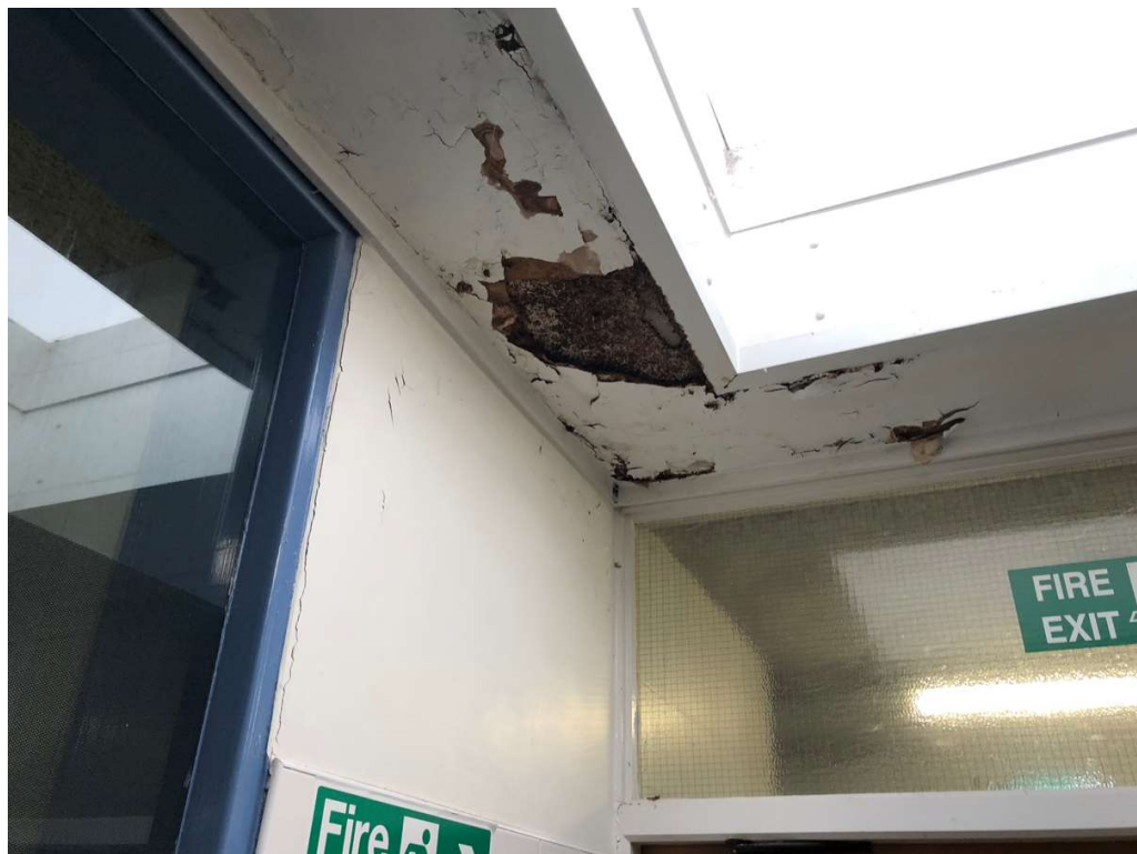
Photo 20: Staining to corridor ceiling due to a leak adjacent to roof light.
