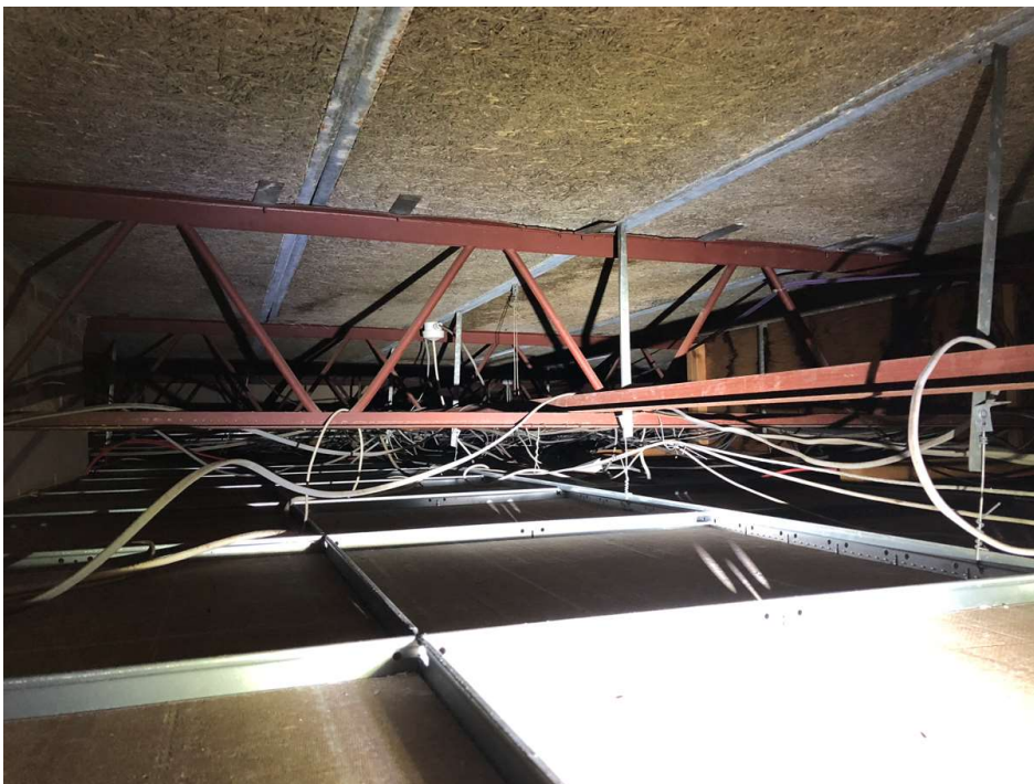
Photo 47: Woodwool roof slabs, bearing onto long-spanning steel lattice trusses. This is above the single storey fitness suite.
