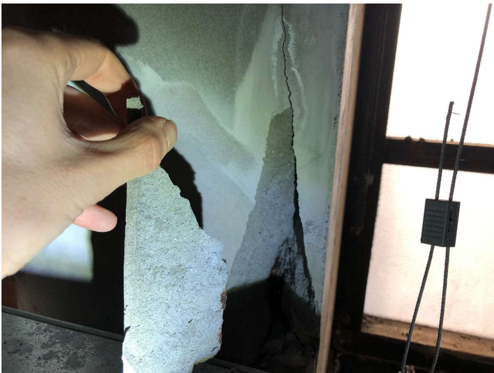
Photo 24: The repair mortar could easily be removed by hand.
