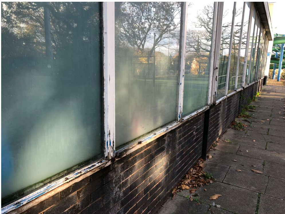
Photo 4: Close-up photo on the rotten frames.
