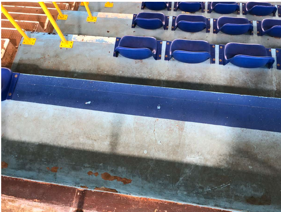
Photo 34: Hairline cracks are visible in the top and to the underside of the concrete tiered seating at mid-span. This is typical to every bay between supporting columns but is not considered structurally significant.
