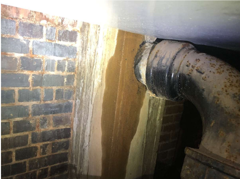
Photo 29: Another example of saturated concrete column on the southwest elevation of the Main Pool building.
