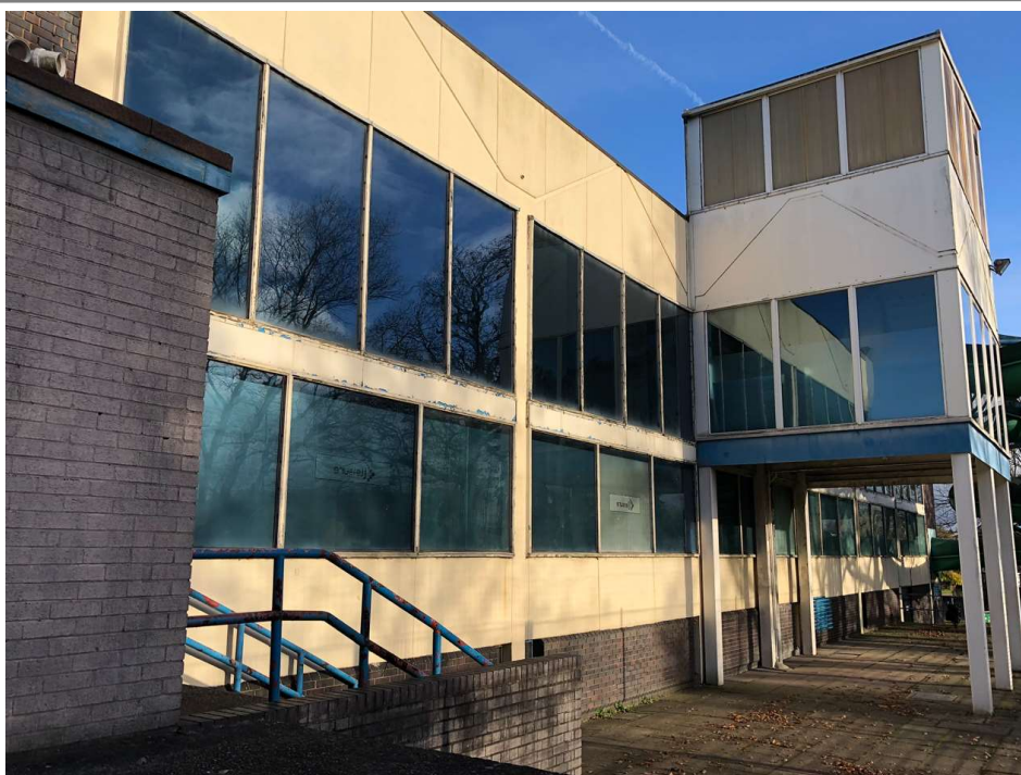
Photo 5: Southwest elevation, Main Pool. The timber framed windows are rotten and require repair or replacement. The two storey frame to the right of the photo is the access to the water slide that is no longer in use.
