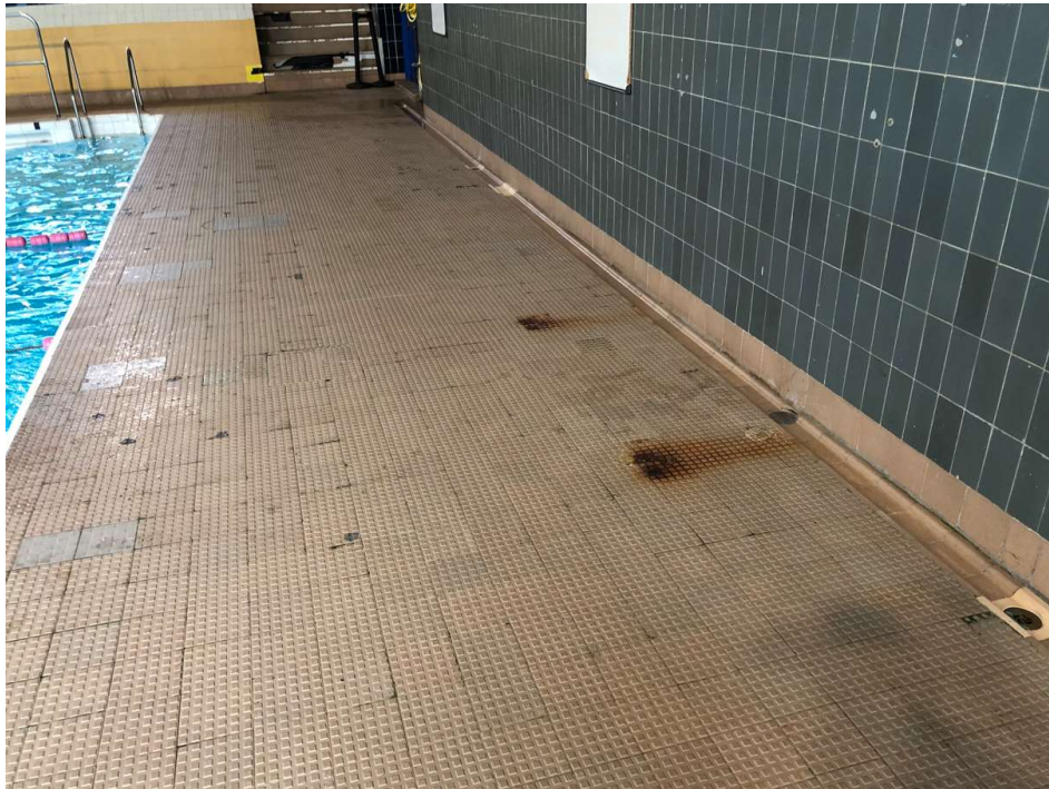
Photo 13: Walkway around the end of the Main Pool. Staining present where corrosion is occurring as the floor is no longer watertight due to equipment having been bolted to the floor. Corrosion mirrored to underside of this floor in the pool basement.
