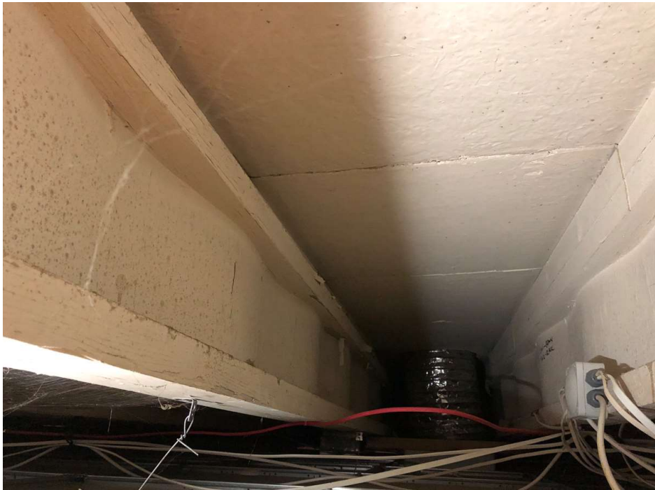
Photo 46: Woodwool roof slabs, painted white, bearing onto long-spanning engineered timber joists. This is above the former squash courts.
