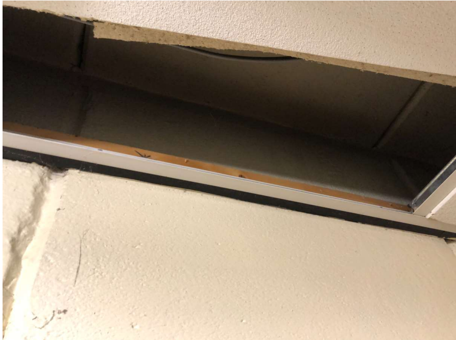
Photo 52: RAAC roof panels bearing onto RAAC wall panels. Photo taken within storeroom at first floor.
