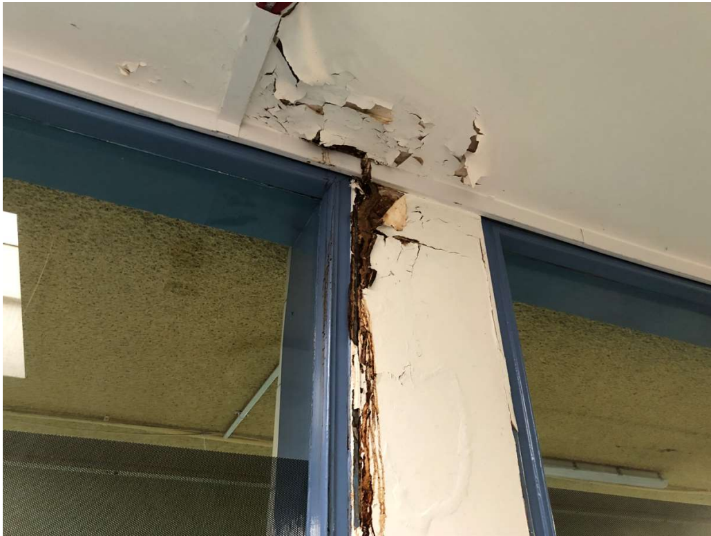
Photo 19: Roof leak causing damage at the top of an internal Teaching Pool column.
