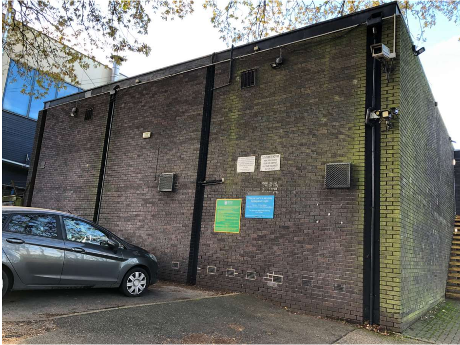
Photo 48: South (end) elevation of RAAC building. Brickwork is in good condition. The roof drains to this end and the RWPs are in recesses within the brickwork. Behind the RWPs are RAAC wall panels painted black. The roof has a small parapet.
