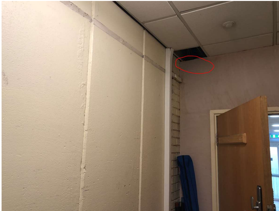
Photo 54: View in storeroom. Vertical RAAC wall panels built in circa 1980 abut the earlier brickwork wall of the 1970s building. The area circled in red is where the RAAC panel has insufficient bearing (photo 53).
