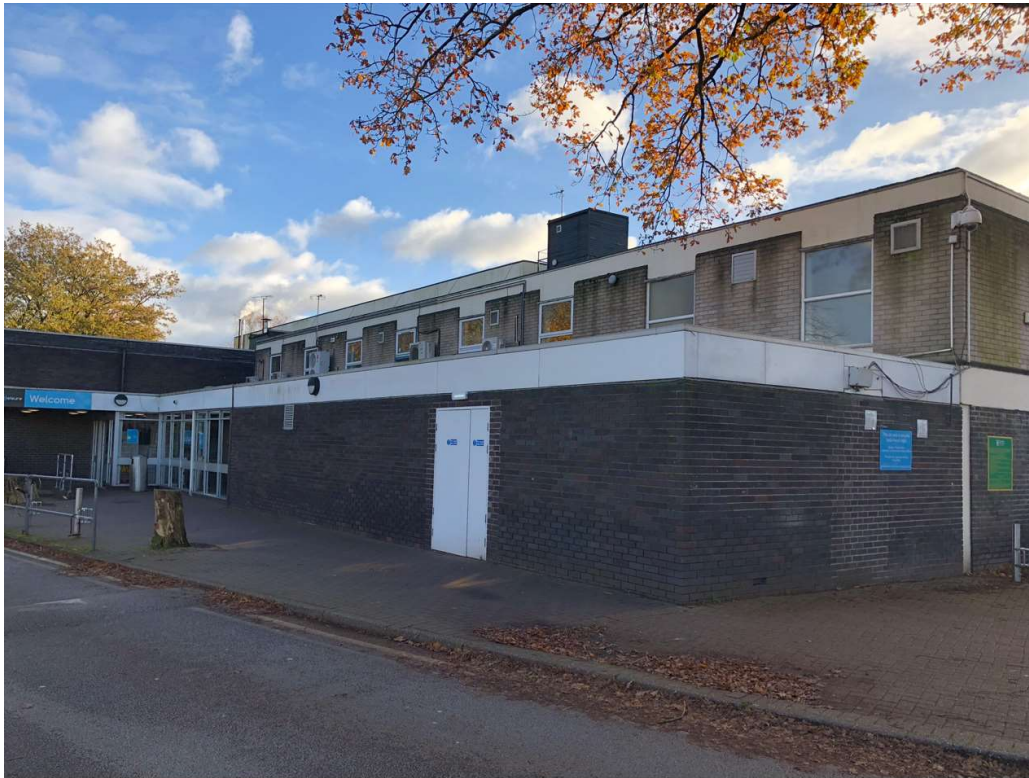
Photo 1: Northeast elevation. Main entrance. Brickwork in reasonable condition.
