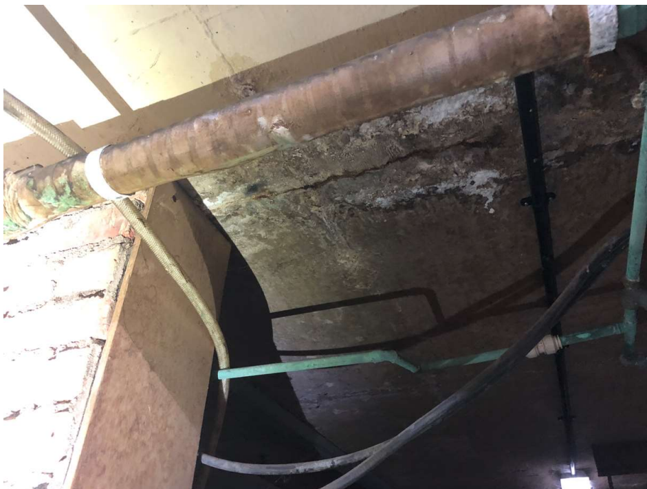
Photo 32: Example of corrosion to underside of floor slab around the swimming pool.
