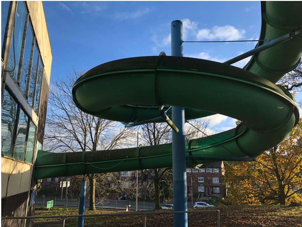
Photo 7: Redundant water slide. Supporting steelwork is in reasonable structural condition.
