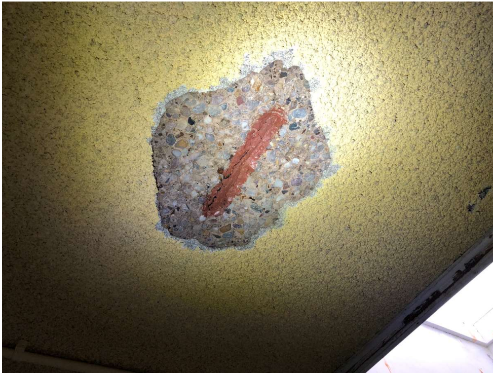
Photo 17: Spalled concrete to the soffit of the Teaching Pool roof. The reinforcement has been coated post-defect to protect it from further corrosion.
