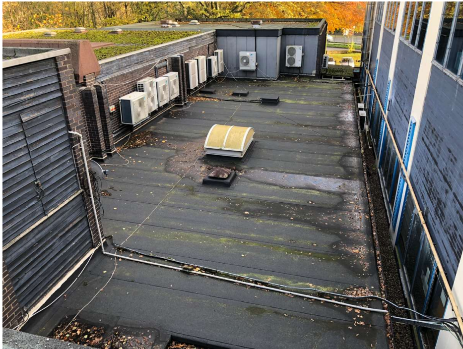
Photo 43: Flat roof over the single storey gym area. The vegetated roof to the left of the photo is above the former squash courts.
