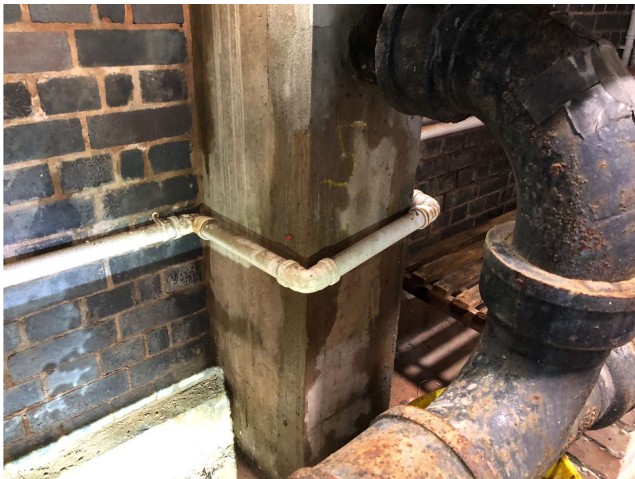
Photo 22: Typical concrete column on the southwest elevation. This column has been previously repaired but is still visibly damp. A drainage pipe, probably a roof RWP, is cast into the column. If this pipe is leaking, which appears to be the case, water will be penetrating deep into the column causing corrosion of the reinforcement.
