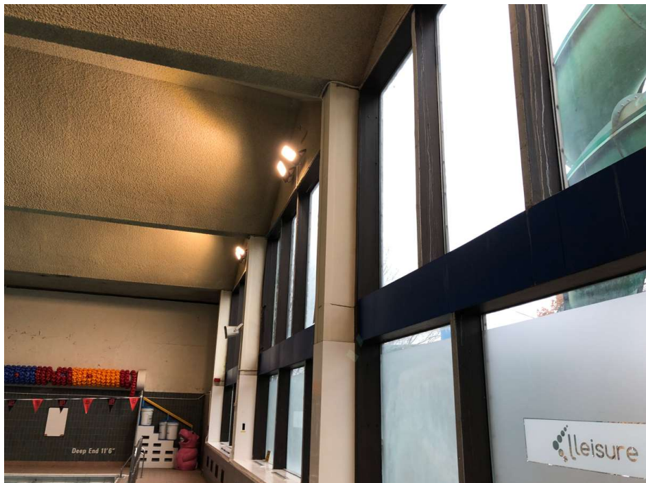
Photo 14: Columns and timber frame curtain walling on southwest elevation. These are the (repaired) columns that have corroded in the pool basement below.
